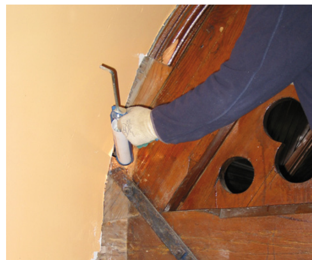
The main truss ends being injected with Tribor Gel which was also used on the wall plates
