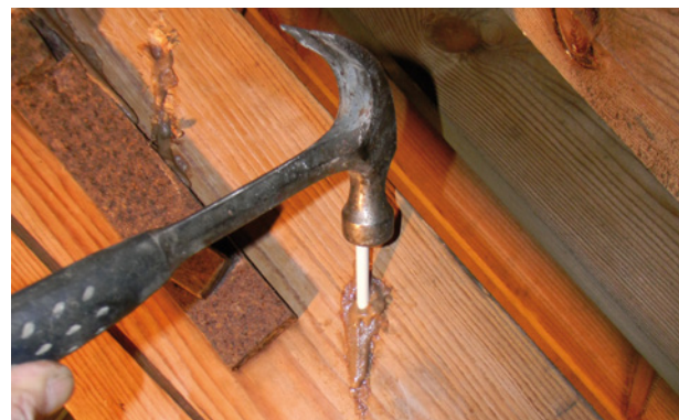
Trimol 50 rods (set in Trimol 36 grout) were hammered in to stitch shakes in main roof trusses
