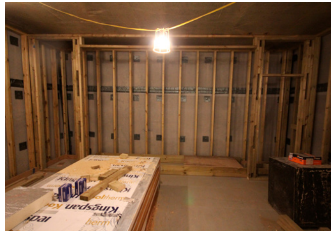
Triton P8 installed behind stud walling
