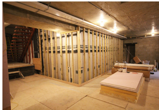
Further Triton P8 installed behind stud walling
