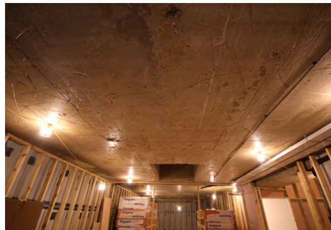
Part of the soffit area using Triton TT Admix in the concrete
