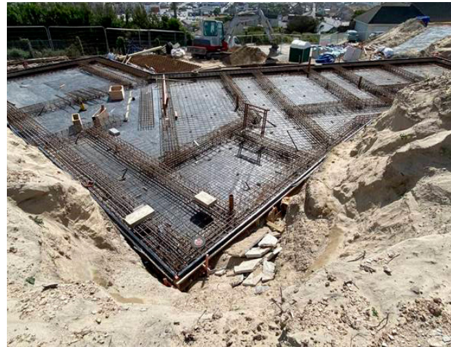
Large slab area ready to be poured in concrete waterproofed by Triton TWS EX-100 membrane.
