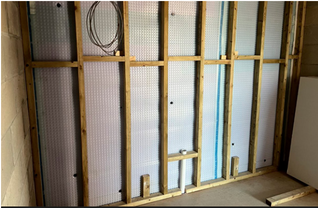
Triton P8 wall membrane with internal timber studwork installed ready for dry lining.
