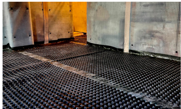
Platon P20 membrane laid to floor, Platon P8 membrane on walls, joints sealed with Platon Cornerstrip
