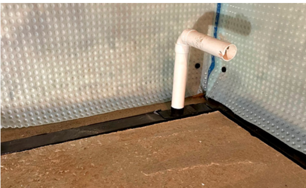
Rodding Eye set in Aquachannel perimeter conduit to allow for future maintenance of system
