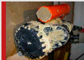
Pump contaminated with free lime
