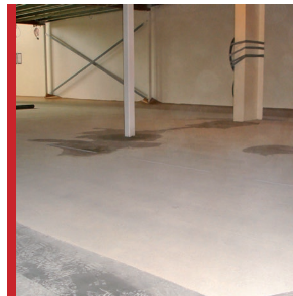
Floor in new build retail unit showing Triton TT Vapour Membrane used as the waterproofing layer, covered with Floor Levelling Compound incorporating Triton LPA/Primer for extra strength.
