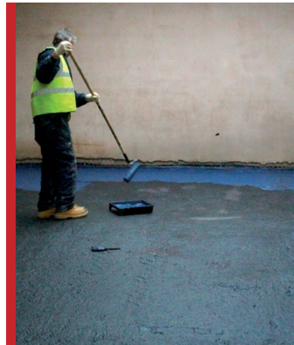
TTVM used in combination with cavity drain membranes to waterproof floor in retrofit basement
