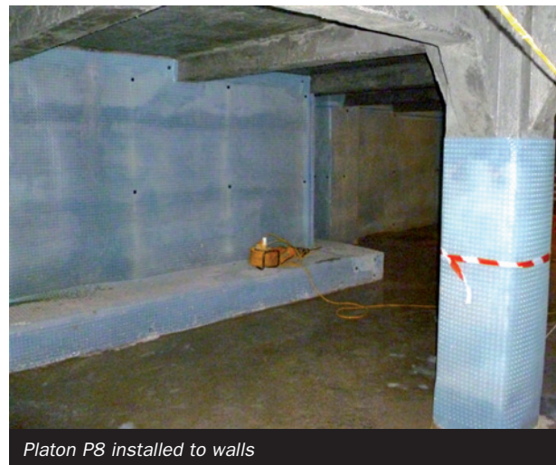
Lime deposits from water ingress
