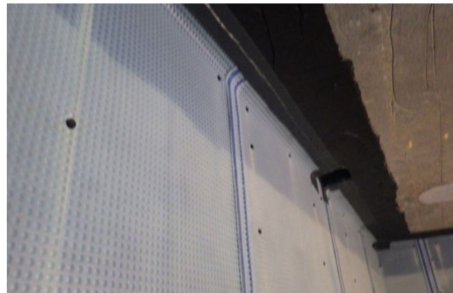
Lower basement level showing Platon P8 membrane on wall to soffit detail sealed with TT Vapour Membrane. 40mm discharge outlets drain down from the level above and angle back towards perimeter liner wall.
