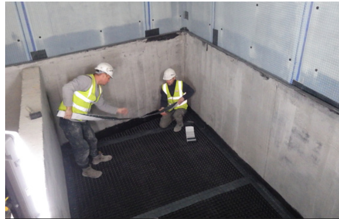
Service trench waterproofed with TT 55 to walls and Platon P20 membrane to floor. Lower basement level drainage channel runs around upstand of trench liner wall and discharges behind wall down to perimeter drainage channel set in trench floor slab.
