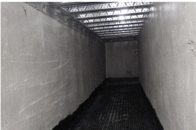
Completed trench looking up to suspended steel floor to lower level basement.
