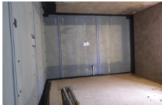
Upper basement level showing P8 membrane to walls and banded perimeter drainage channel.
