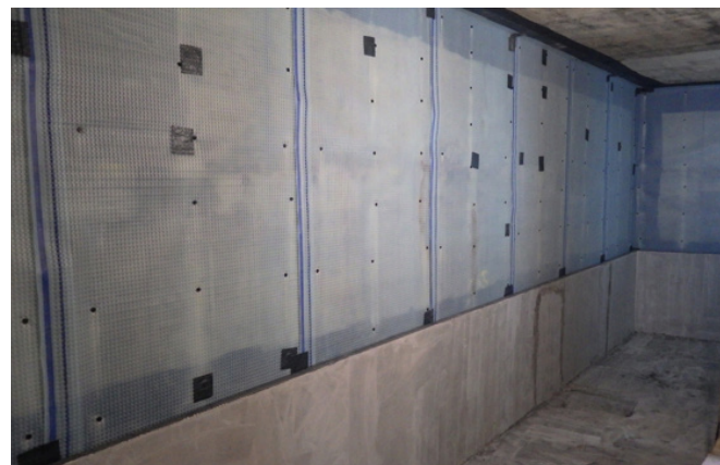
Swimming pool recessed into lower basement level floor. Perimeter drainage channel at floor level runs around top of pool liner wall. Pool walls and floors are waterproofed with TT55/TTME with Fillet Seal detail at wall/floor joints.
