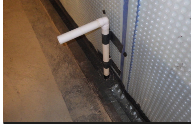
Platon P8 membrane to wall at upper basement level with perimeter drainage channel sealed with TT Vapour Membrane and Corner Strip, showing access point via 40mm pipe and 90° bend.
