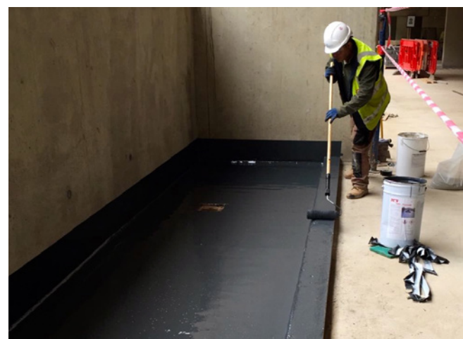
Two coats of TWS Fastcoat provided an impervious barrier to the subterranean floor slabs
