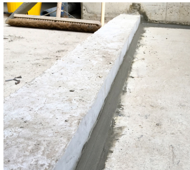
Triton Fillet Seal was applied to eliminate 90° angles at wall floor transitions and minimise risk of leaving gaps or holes unsealed
