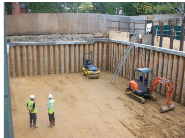
After dig out, a sand bed was applied over crushed concrete before application of 50mm layer of blinding concrete
