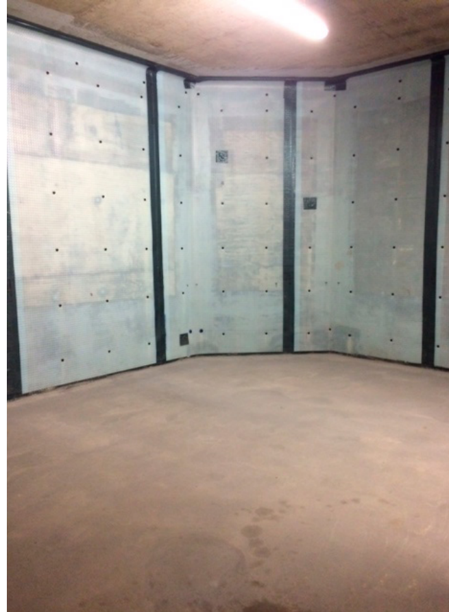
Platon P8 to walls fastened with Brick Plugs and Platon Corner Strip sealing joints following screed to Platon P20 on floor
