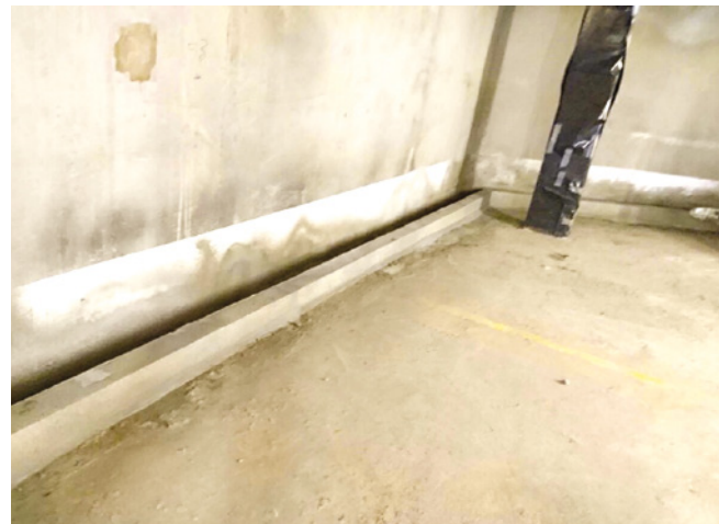
Concrete upstand created to form gully for Aqua Channel for perimeter cavity drain membrane system
